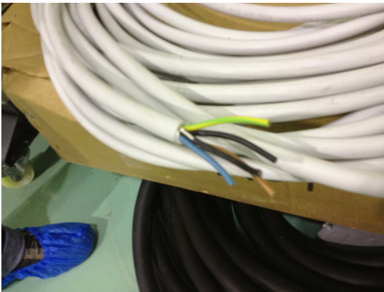
(Figure 1) These wires contained in the high voltage power cables are used to power most of the Virgo infrastructure. Three of the cables are used to transmit the three-phase current while the fourth acts as a “neutral” wire sending a reverse current whose amplitude in time is the sum of the three phases while a fifth wire acts as ground.
