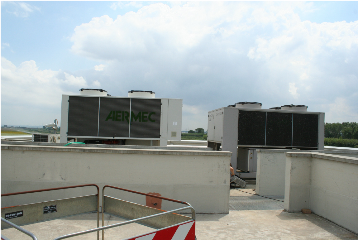
Figure 12 - The two water chillers (Number 2 (old) on the right, Number 1 (new) on the left) on the TechBuilding roof.
